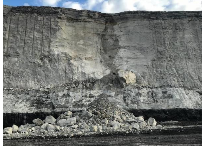
Figure 8 Case study 3, post failure slope conditions
